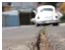
Inhabitant of the Izcalli District in the center of Ecatepec municipality – State of Mexico (Valley of Cuautitlan-Texcoco) complain about the deterioration of the highways caused by the natural gas network which has been constructed by the Mexigas Company. © Newspaper El Universal (Mexico) - Photographic Archives / Photographer: Luis Garcia Soto
